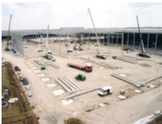
Erection taking place on four work fronts, with steel lay down areas for each gang
