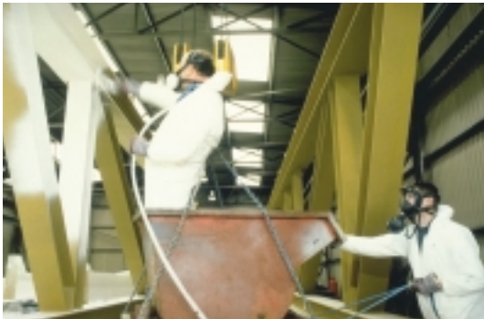
Off-site intumescent coatings are applied manually in large, heated sheds with good air movement
