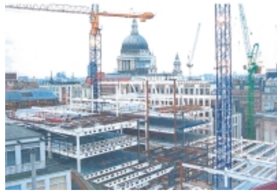
10 Gresham Street has 18 m clear span floors throughout, with all service penetrations through the beams with large over-provision for change.
