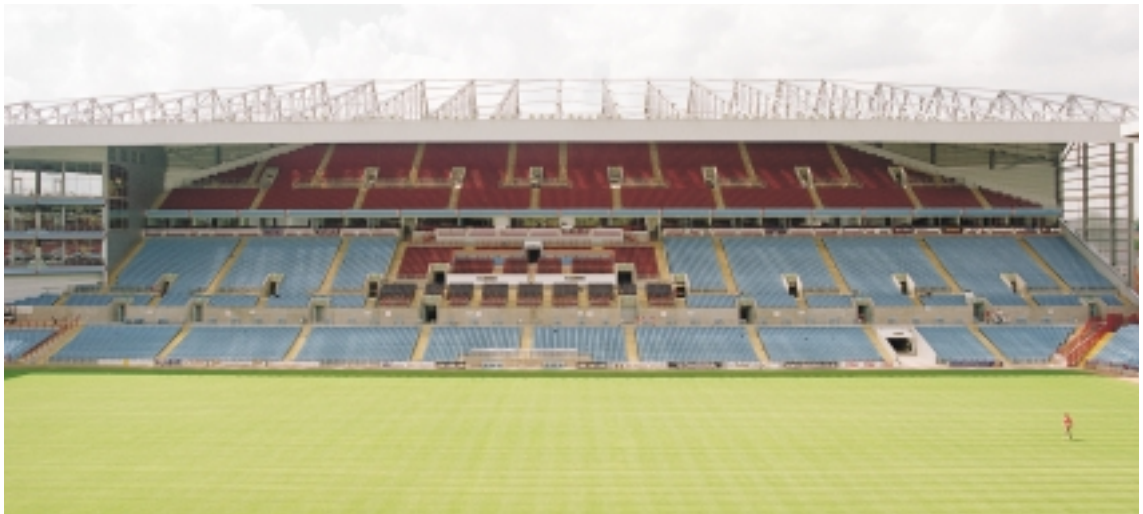
Category M Steelwork - The New Trinity Road Stand, Aston Villa Football Club – James Killelea & Co Ltd
