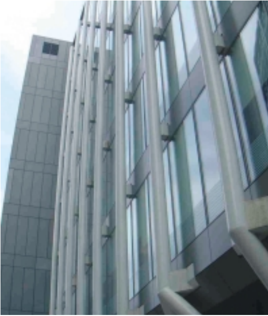
Fleet Place, Holborn with simple rectangular spigots penetrating cladding with joint to floor beams inside the cladding.
