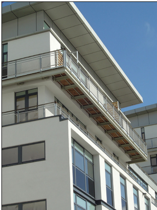
Figure 3.4 Details of insulated render cladding at parapet and balcony - Cala House, Glasgow
