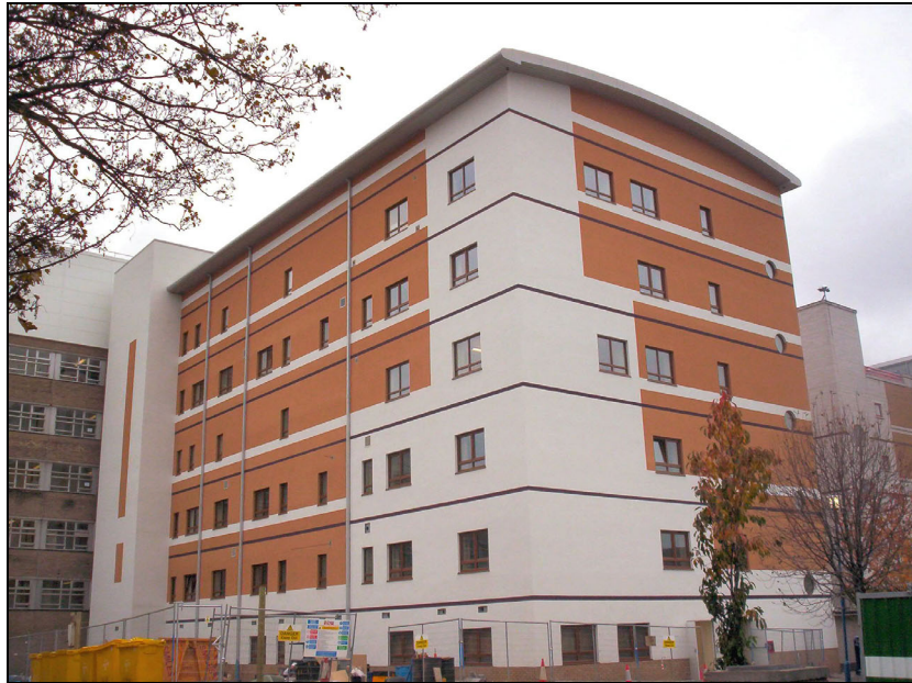
Figure 3.5 Insulated render used in multi-storey building at Sunderland Royal Hospital showing detailing at floor lines
