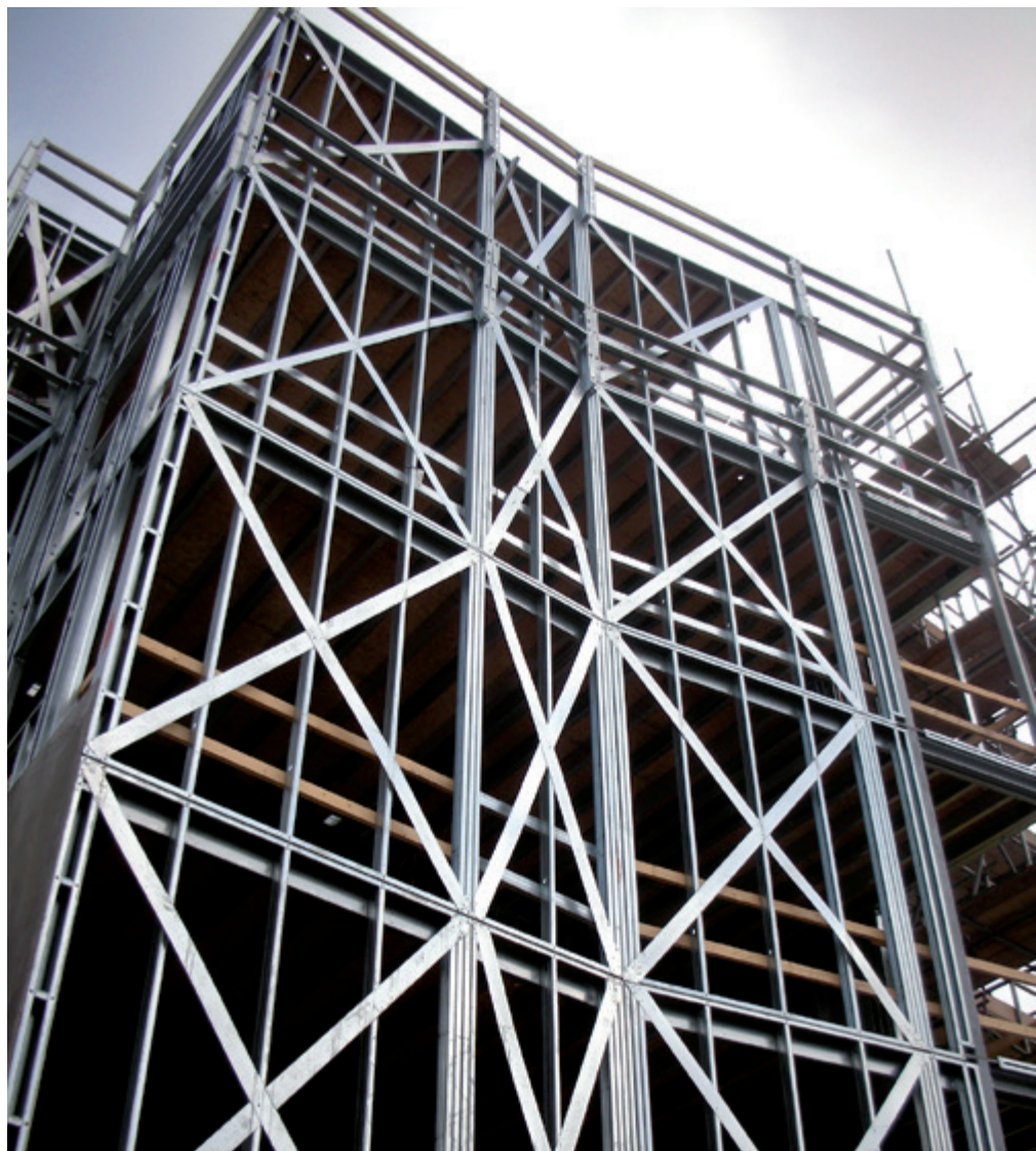
Figure 2.2 X braced frames in a multi-storey building (Photo courtesy of Metek UK Ltd.)
