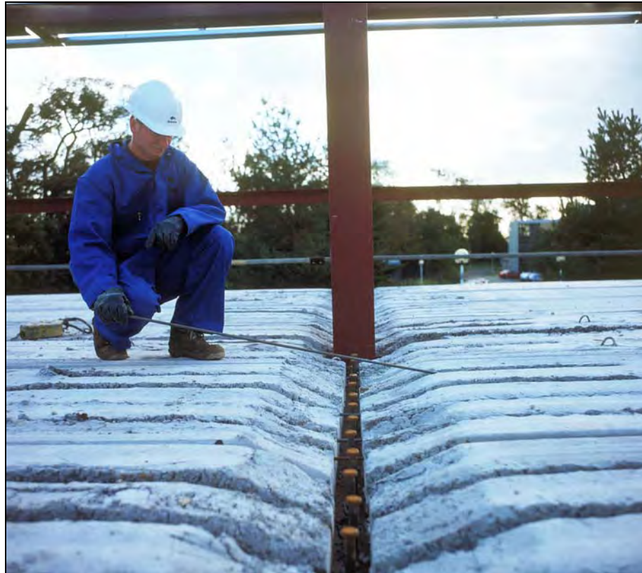
Figure 5.12 Composite floor construction with precast concrete hollow core units, showing transverse reinforcement bars placed within open cores
