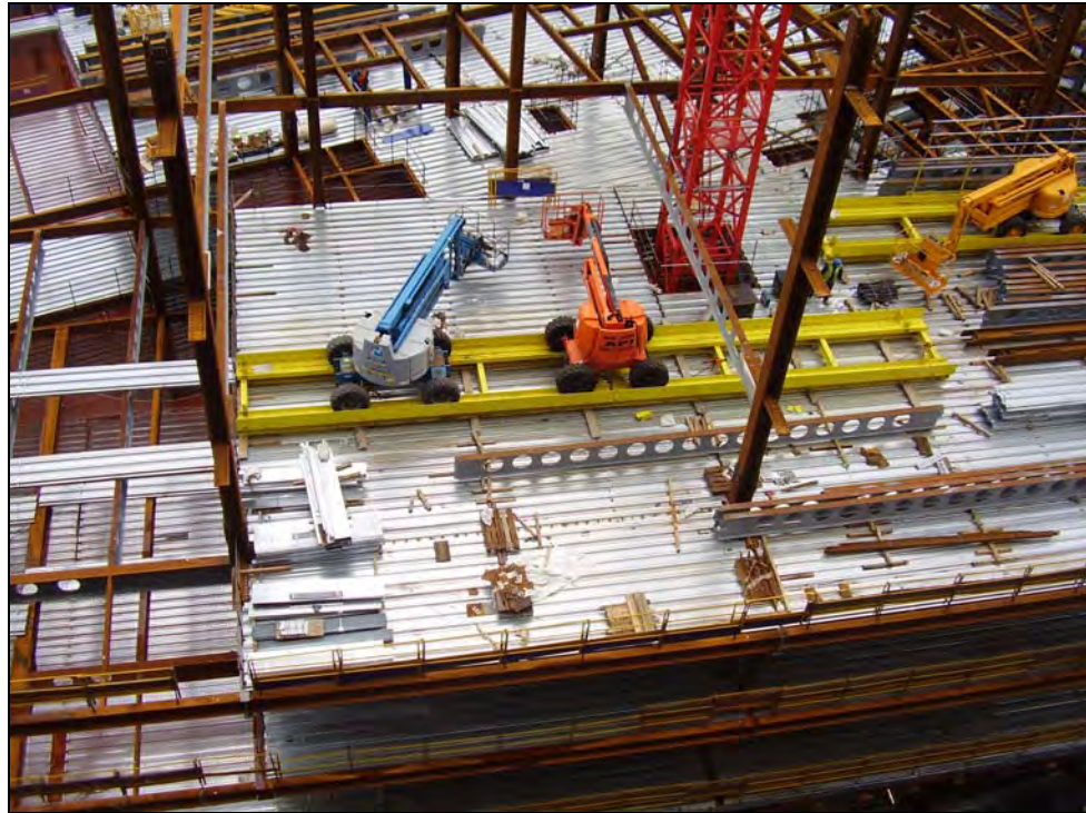
Figure 2.2 Rapid, safe installation of steelwork and steel decking from a mobile erection platform speeds up the construction process
