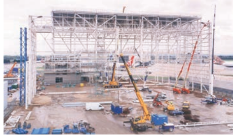
Roof steelwork assembled at low level and lifted to height using jacking towers
