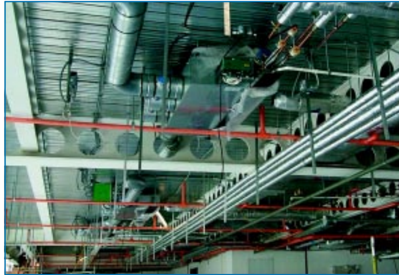
Figure 17: While this installation shows the integration of services with structure, deviations laterally and horizontally hint at a sequential rather than a truly integrated design process. ©BSRIA.
