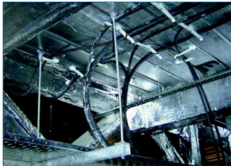
Figure 22: Between 40 to 60 mm of depth can be lost from the underside of the slab to the bottom face of a ceiling, adversely affecting the ability to run cabling horizontally. ©BSRIA.
