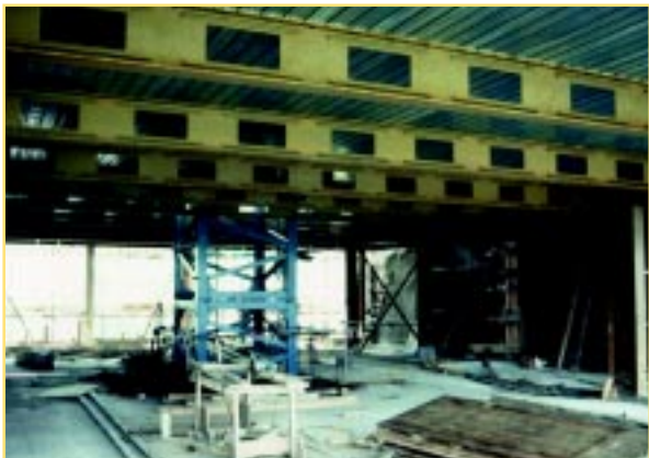
4 Figure 7: A standard universal beam cut with rectangular apertures. A symmetrical layout such as this gives wide scope for services distribution, though not necessarily optimal. Note the horizontal stiffeners above and below the openings. ©SCI.
