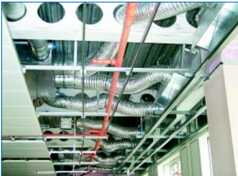
Figure 24: An uncontrolled number of bends in flexible ductwork will cause loss of self-balancing between diffusers, and added noise through the diffuser that gets more air. ©BSRIA.
