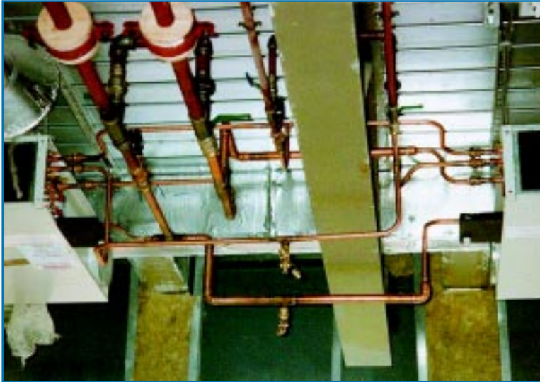
Figure 19: More poor services-to-beam interface engineering. The fitting of drain cocks and valves such as these could not only interfere with other services such as light fittings, they could be low enough to foul the suspended ceiling. ©BSRIA.
