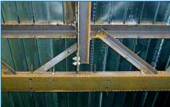
3 Figure 6: A typical lattice girder prior to the application of fire protection. ©BSRIA.
