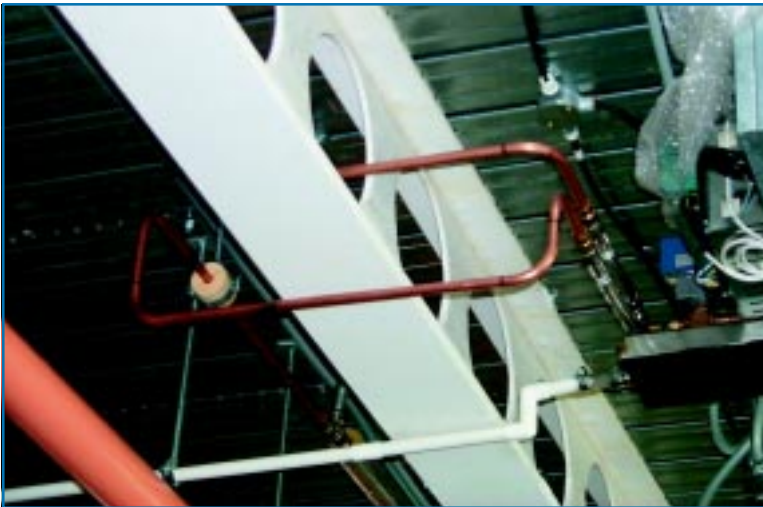
Figure 20: Poor interface engineering between a cellular beam and a fan-coil unit. The condensate pipework has been forced to deviate immediately after leaving the fan coil unit. More attention at the design stage could have avoided this problem. ©BSRIA.
