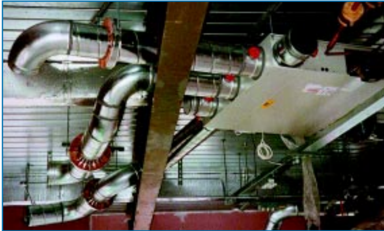
Figure 23: The use of rigid ventilation ductwork fed through beams can result in a high number of deviation pieces, all of which are labour-intensive to fabricate and fit, and as a consequence be a source of air leaks during building operation. ©BSRIA.
