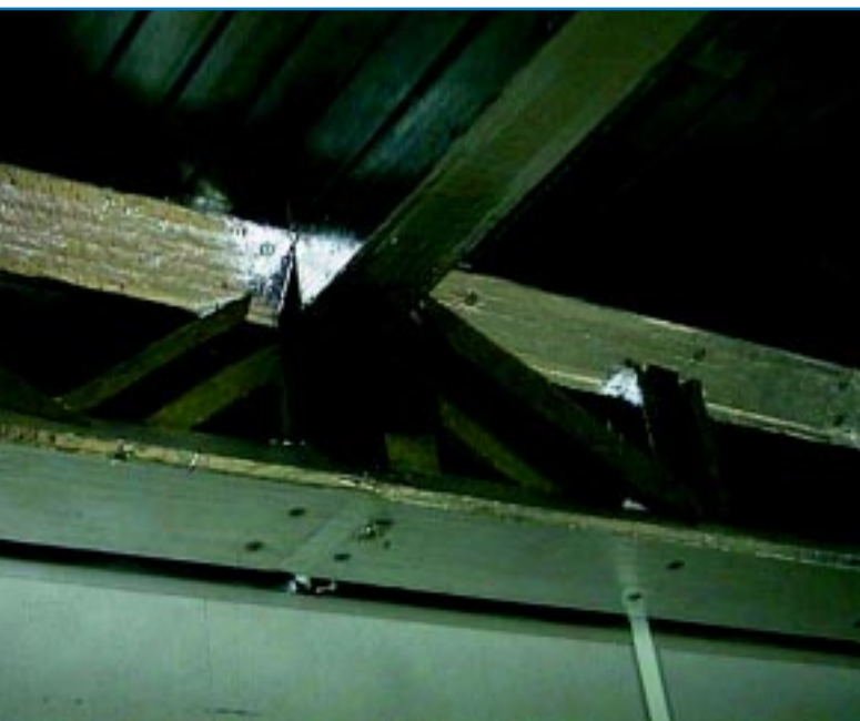
Above, figure 16: A lattice beam enclosed by a fibreboard-based fire protection system. Note that the free area of the beam is now considerably reduced. ©BSRIA.
