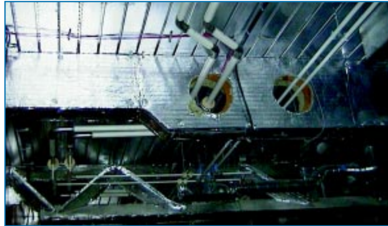
Figure 21: A contractor's attempt to co-ordinate services through a cellular beam and a lattice-web beam. Note the number of deviations necessary for the services to pass through the beams. ©BSRIA.
