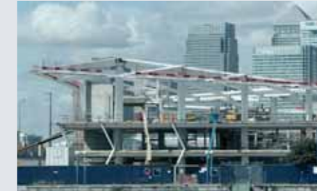
The roof cantilevers up to 15m from the grid of steel columns.
