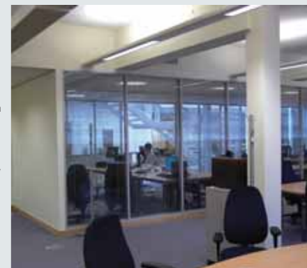
The steel-framed building has a hollow core deck with an exposed concrete soffit.
