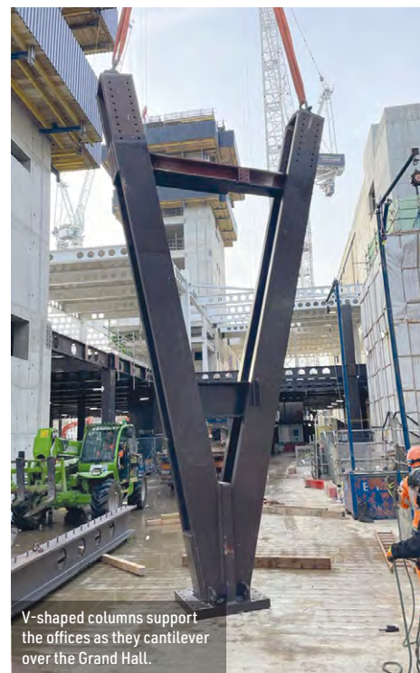
Steelwork is erected to form the rooftop sky garden and (right), the grillage to support the hotel commences.
