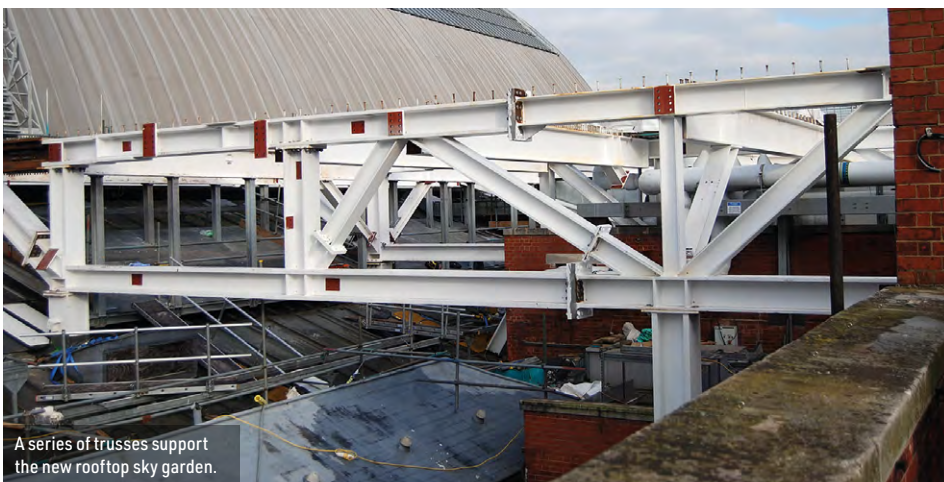
New trusses span the existing exhibition space and support the West Hall's second and third floor venue.
