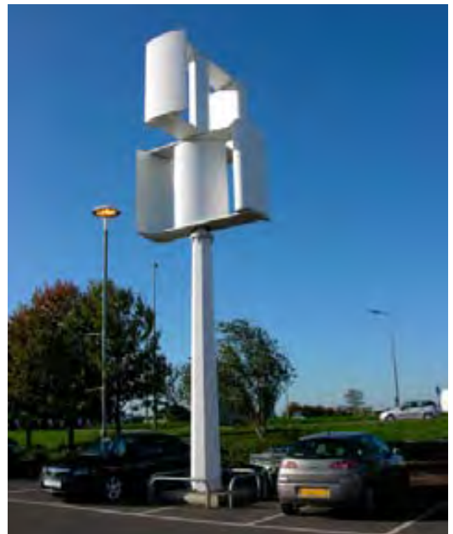
ON-SITE WIND TURBINE
