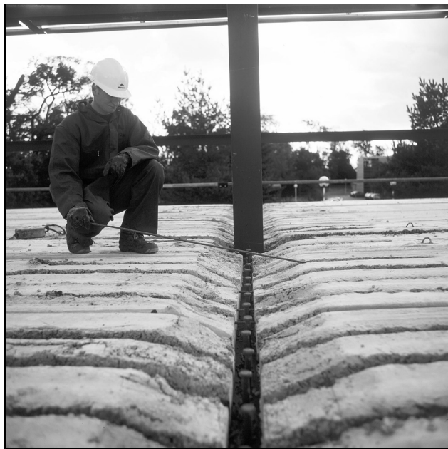
Figure 5.14 composite floor construction with precast concrete hollow core units, showing transverse reinforcement bars placed within open cores
