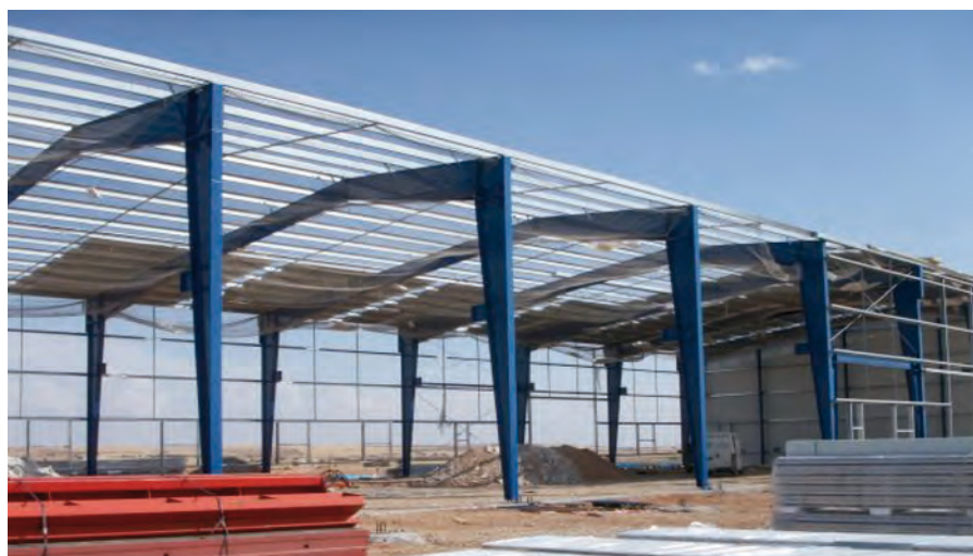
Figure 5.9 Single portal frames with tapered columns and rafters under construction in Spain
