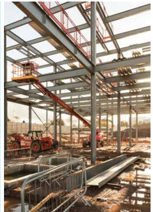
Above: An aerial view of the Longbridge site, Birmingham Opposite and this image: Construction work taking place at Longbridge towards the end of 2014
