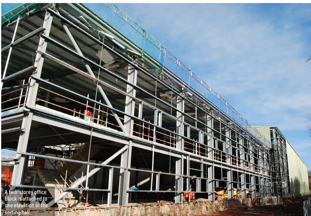
To allow easier truck movements in the completed scheme, a roof level truss allows the reception hall to have a large column-free space.
