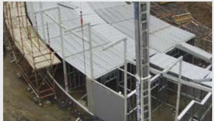
Multi-storey light steel framing with some hot rolled steel members. Courtesy, Fusion Building Systems.
