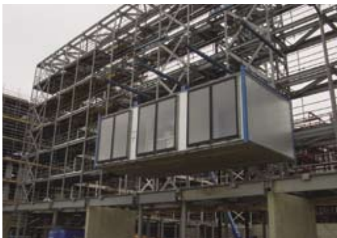
Modules delivered 'just in time' to site in Manchester. Courtesy, Yorkon and ShedKM Architects.
