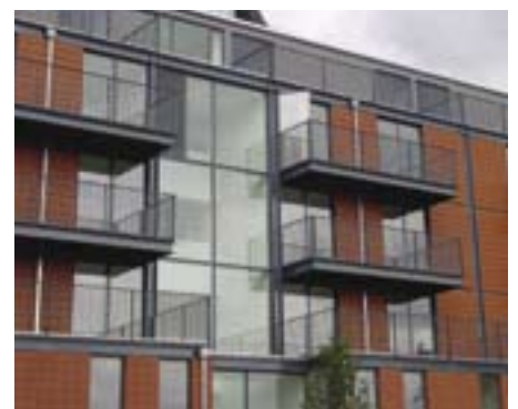
Mixed modular and light steel framing in a social housing project. Courtesy, Feilden Clegg Bradley.
