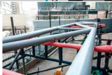
One of the atria's trusses is assembled before being lifted into place
