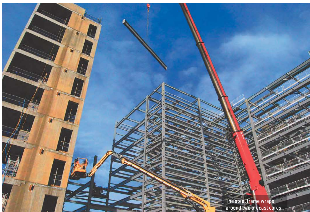
The completed structure will have a living wall covering each core and a series of plant boxes on the southern facade.
