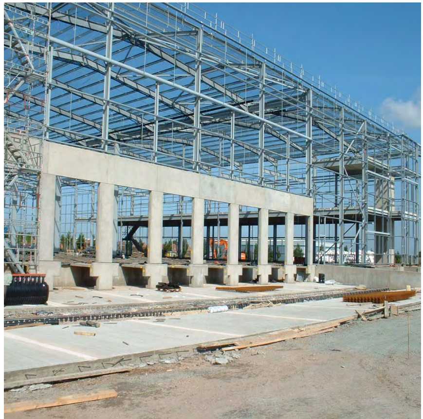
Precast loading docks, Prologis Park, Coventry Courtesy of Barrett Steel Buildings Ltd
