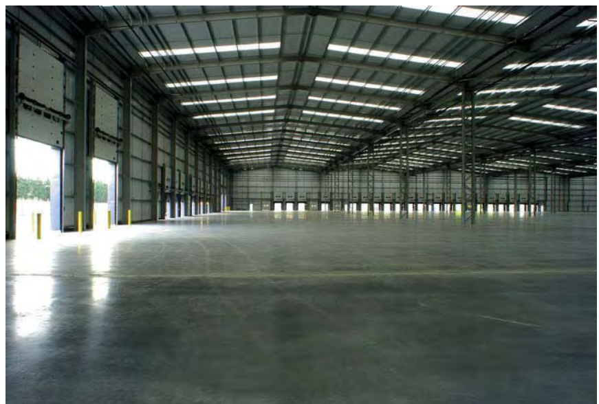
Concrete slab in a typical distribution warehouse Courtesy of Michael Sparks Associates
