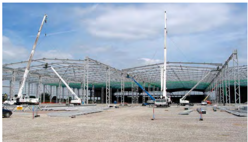
Distribution warehouse for Argos Direct, Bedford Courtesy of Barrett Steel Buildings Ltd.
