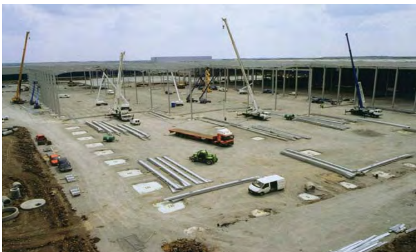
Steel erection in progress at TNT FastTrack, Lutterworth Courtesy of Barrett Steel Buildings Ltd
