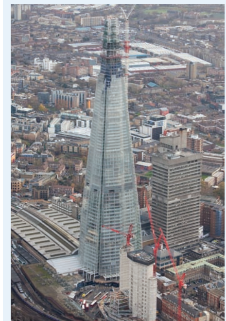
At 310m the Shard will be the tallest building in the EU when it completes later this year.
