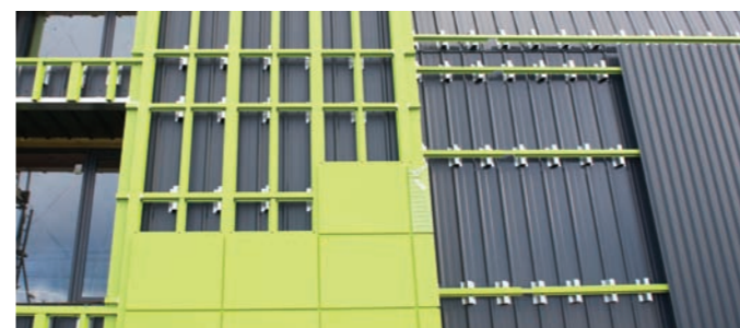
The Linden Green cassette facade system (left) was installed to part of the SBEC building to heat the offices, while the Anthracite collectors (right) feed pre-heated air into the prototyping bay.
